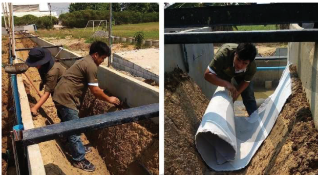
Figure 2b Building up simulative ditch by clay and lining with concrete fabric
