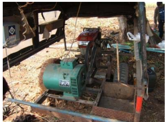
Figure 2 Electric generator for Submersible pump.
