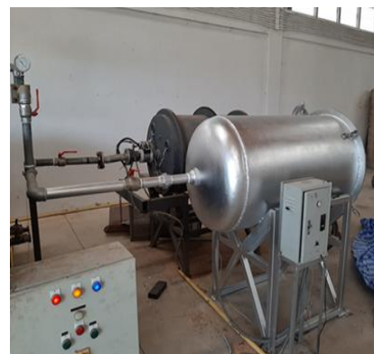
Figure 11 Assembly machine and Equipment
